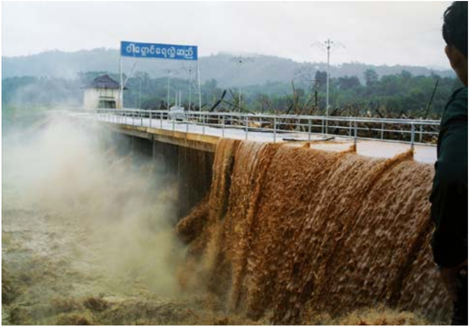
The Washawng Dam in Kachin State breaking in May 2006; the resulting flood completely destroyed the dam
