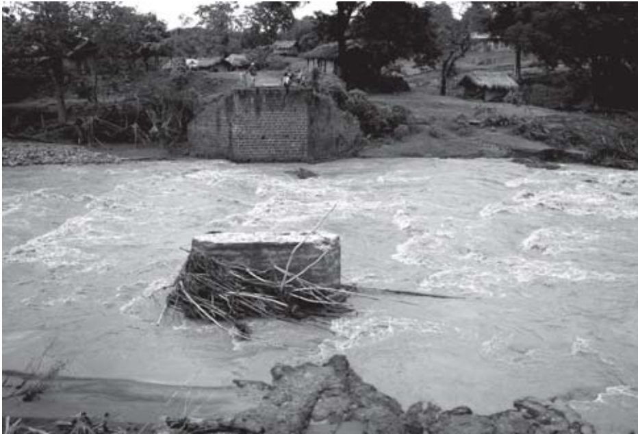
All that remains of the Ching Hkrang Dam after it was destroyed in a flood
